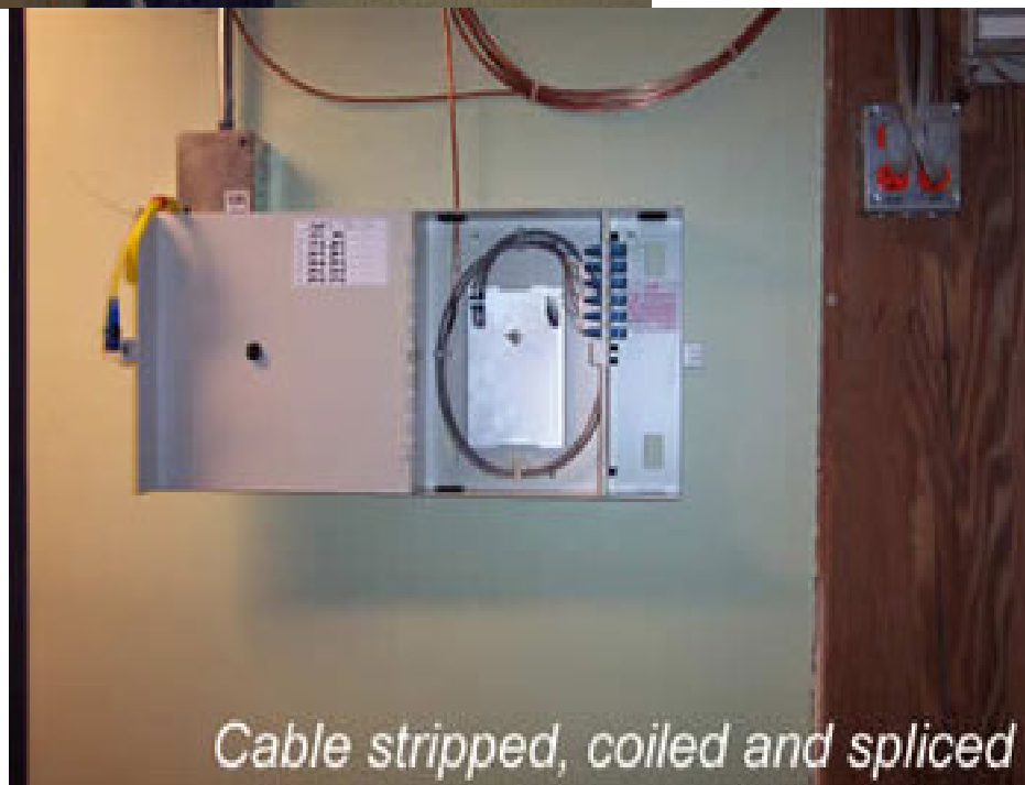
Server room installation
